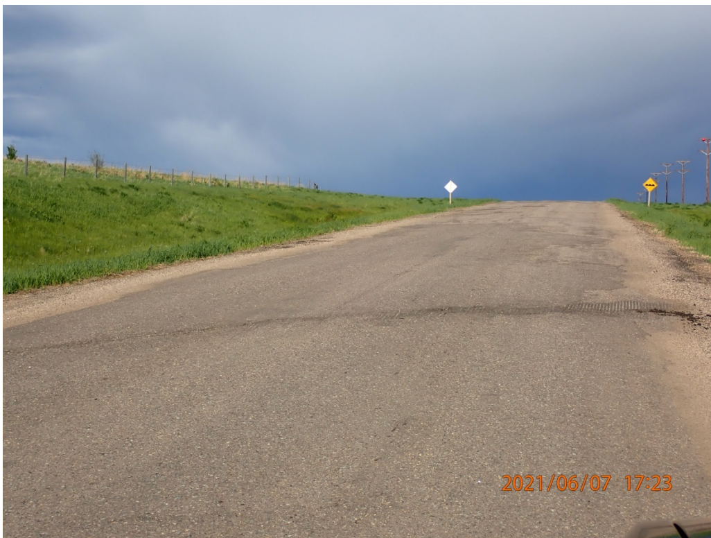
Photograph 2: East slope middle crack
